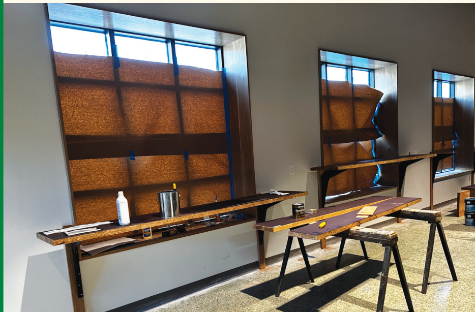
Our bar seating area at the front windows which is currently under construction.
