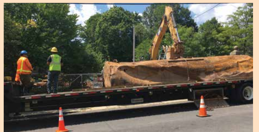
Workers from Kleinfelder Engineers secure the old oil tank to a flatbed truck
