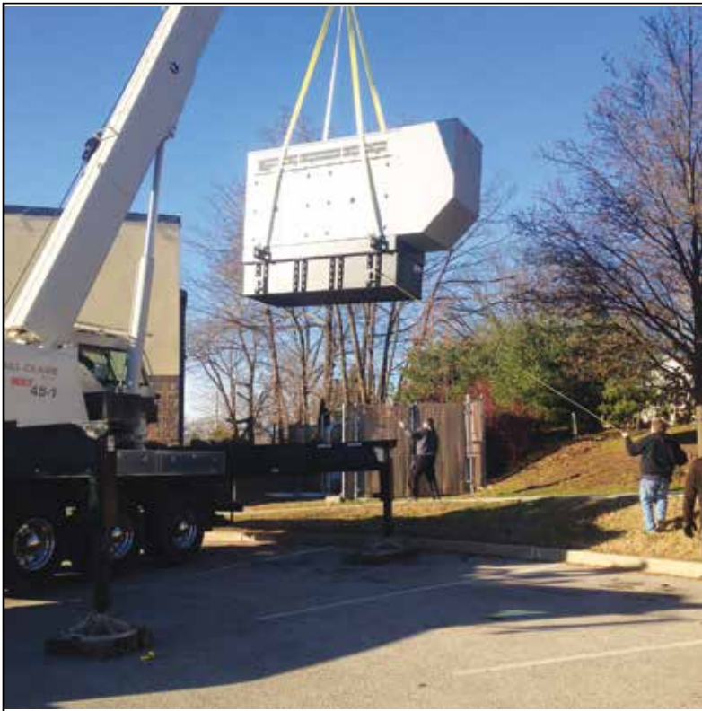
Workers hoist a new backup generator onto the roof of our Ambler store. The new backup can be fired up in the event of a power failure, ensuring that the lights, registers and refrigeration can all stay on.
